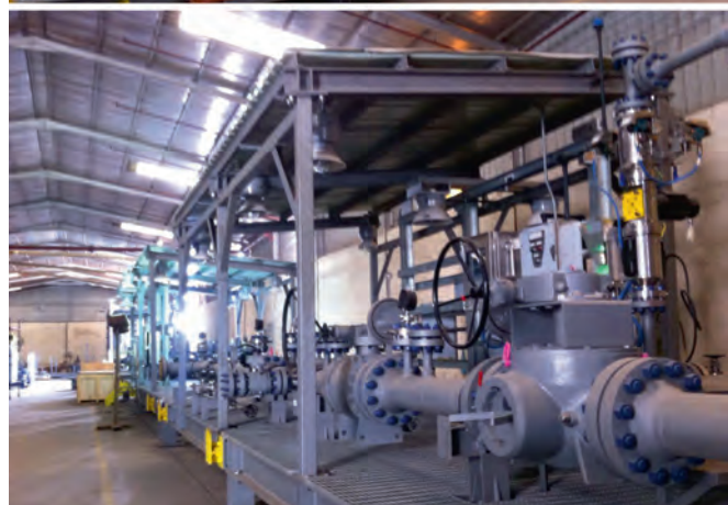
AES has state-of-the-art facilities in Saudi Arabia to build and commission water desalination plants and modular skids
