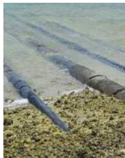
Pipeline in an intertidal zone
