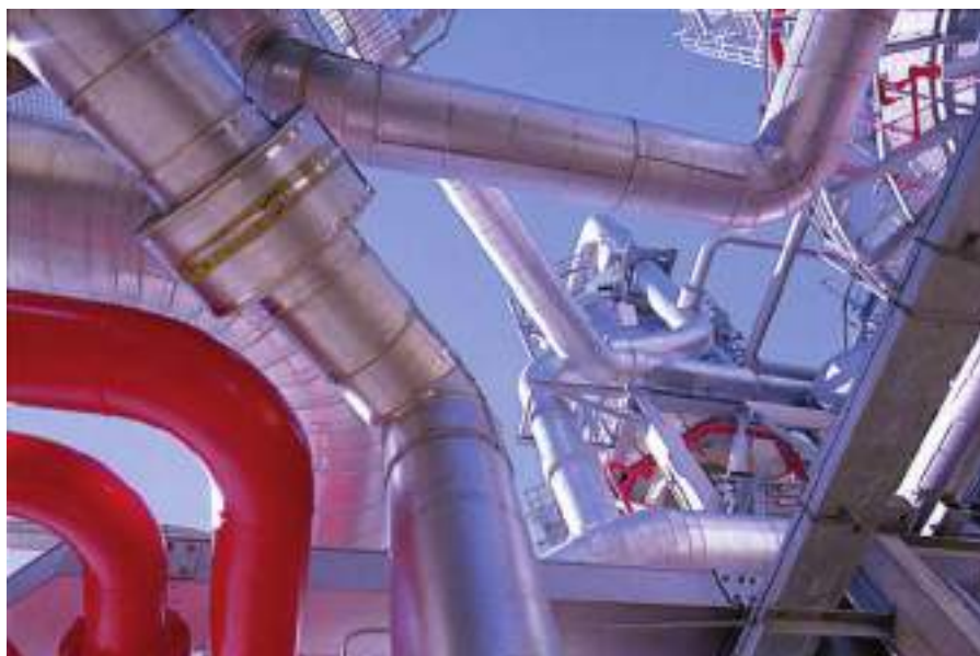
The industry's operating environments can restrict the functionality of wireless systems (Photo: BP plc)
